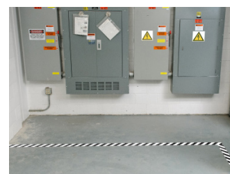
6. Colour-code areas in front of electrical panels.
