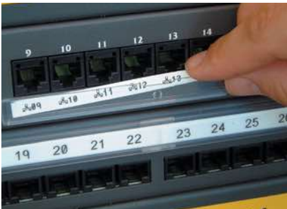
Punch block & patch panel labels
