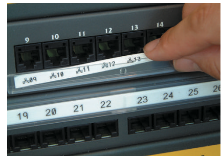
Punch block & patch panel labels
